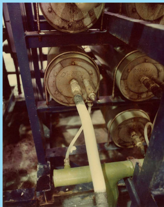
Southwest Plant 1 DOWEX Hollow Fiber RO Permeators installed in 1977
