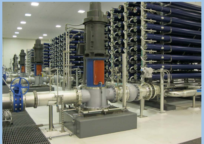
North RO Plant Production Trains and High Pressure Pumps
