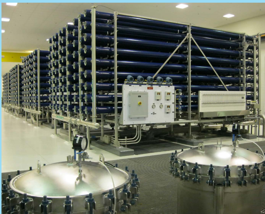
North RO Plant Cartridge Filters and Production Trains
