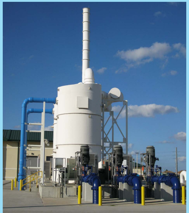
Clearwell Transfer Pumps, Degasifiers, and Dispersion Tower
