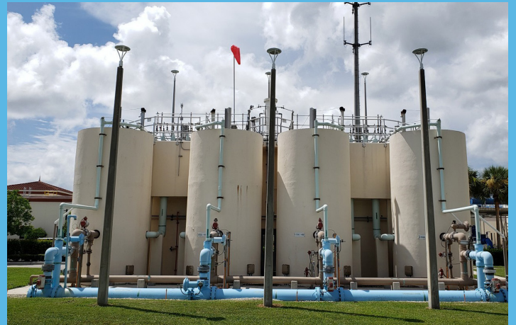
Ion Exchange Plant
