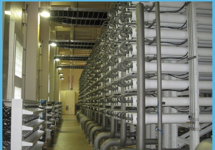
14.5 MGD Nanofiltration Trains
